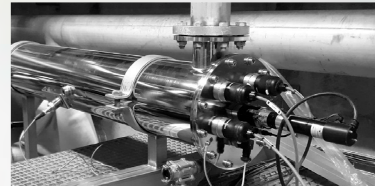
Installed MR3-220SSV in Porvoo Finland
